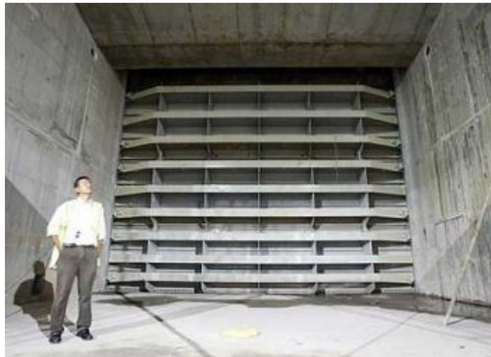
Key gate: The flood gate which channels water to the Taman Desa holding pond.
