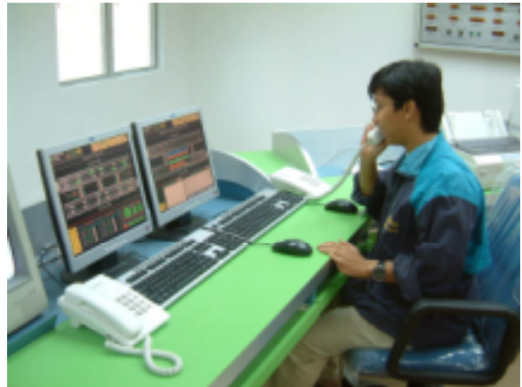
Figure-2: Local TCMS Control Room
